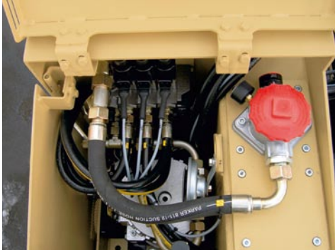
Service access hydraulic system
